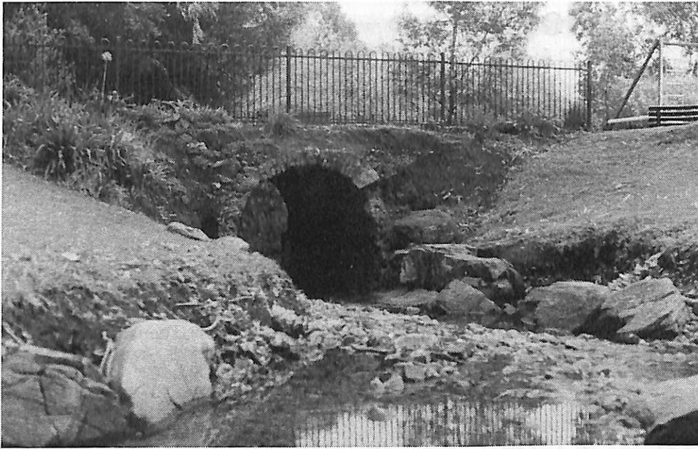
An early bridge over First Creek at the end of Bond Street, Norwood.
