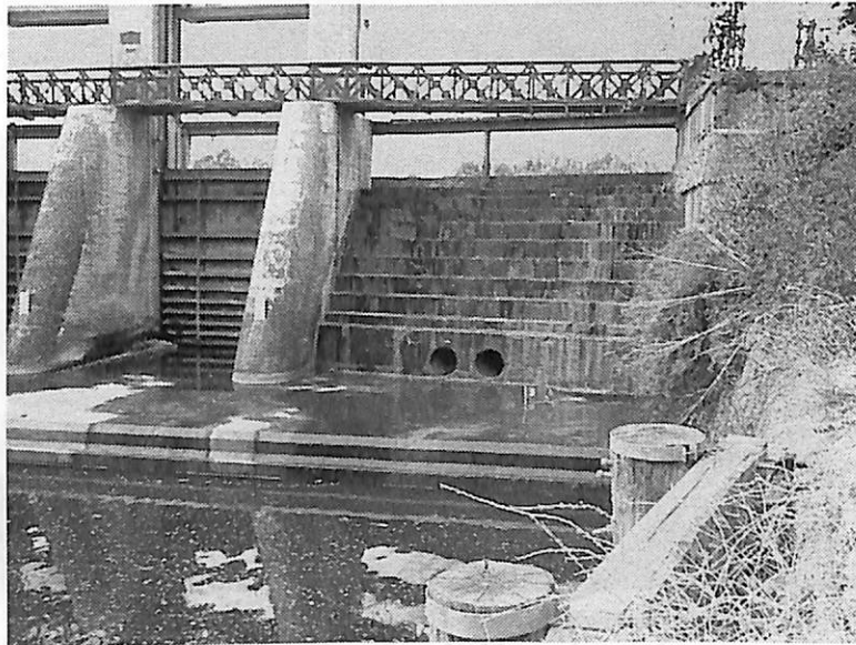
The present weir on the Torrens. Two of the original circular sluice gates can be seen in the centre of the photograph.
