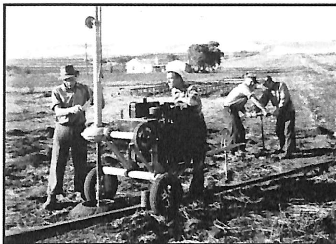
Preparing footings for pre-fabricated houses in the Marion district, early 1950s. From left; Heinz Schoemann, bricklayer; Guenther Diesing, labourer; Horst Eisenbach, plumber; and Heinz Schmitz, joiner-carpenter.
