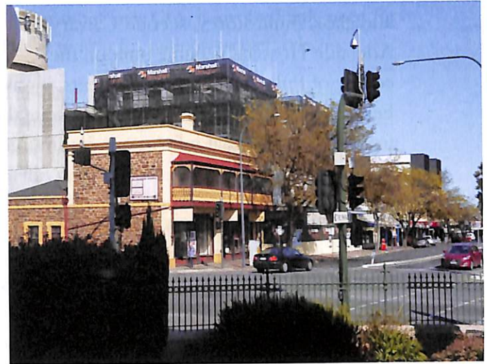
Eastern end of Norwood Parade as seen from the front steps of Clayton Wesley Uniting Church showing two high-rise buildings currently under construction. The intersection of Portrush Road and The Parade has three State Heritage-listed buildings.
